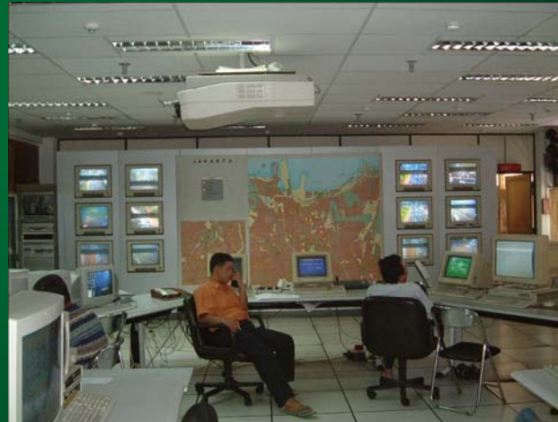
Area Traffic Control System
